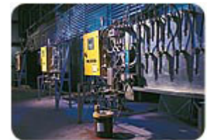
The fluid meters and valves work together to control the flow of the individual materials to the systems integrator.
